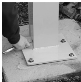
Figure 4.5 Bolt Down Raceway
